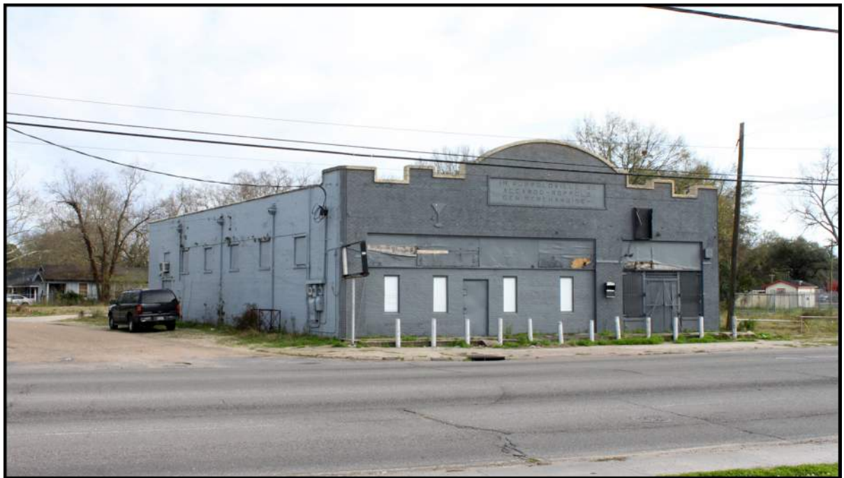
Figure 4-24. The windows have been enclosed and/or boarded. View is to the southeast.
