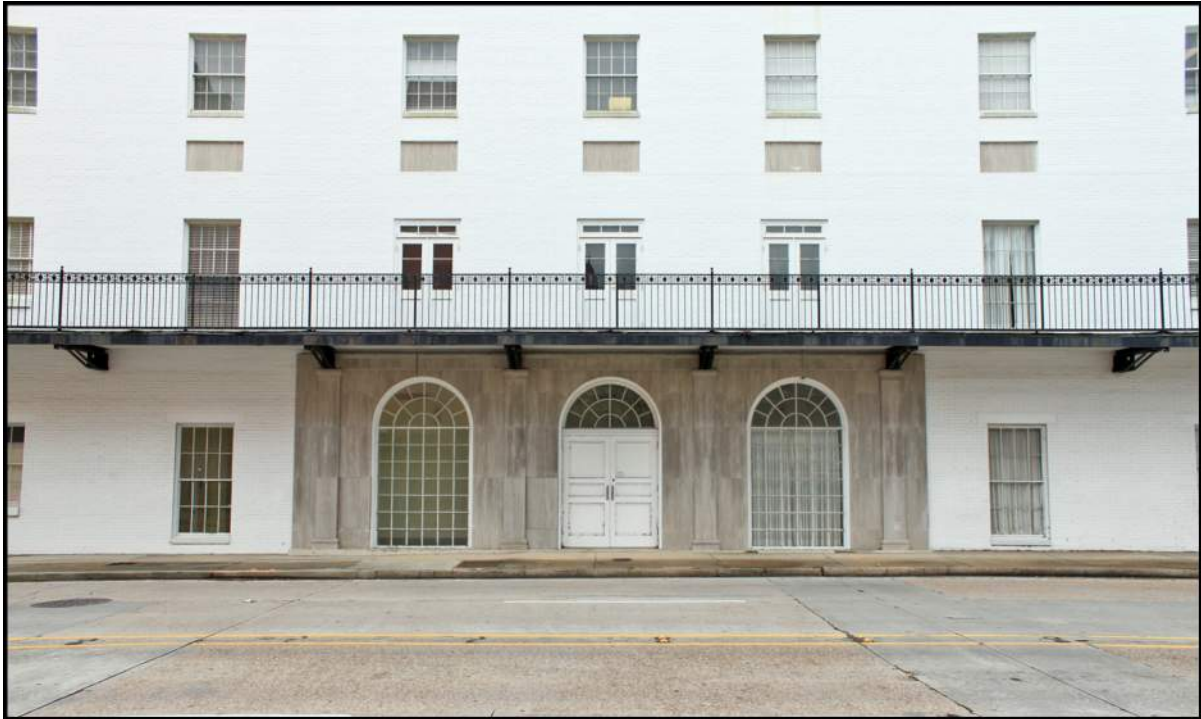
Figure 4-18. The Florida Street entrance has a marble surround on the first floor, a wrought-iron balcony on the second, and a series of marble panels between the second and third floors. View is to the south.
