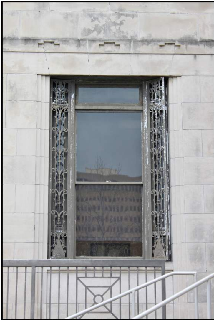
Figure 4-8. The original 2/2 windows have been replaced with 1/1s, but the original surrounds and frames remain intact.
